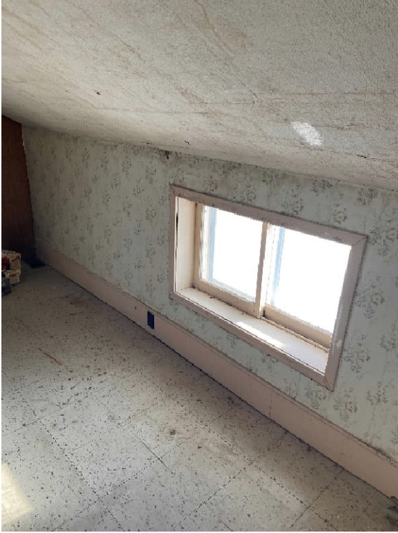
Plate 56: Detail of east knee wall or "bellyflop" window with recent trim in the northeast room
