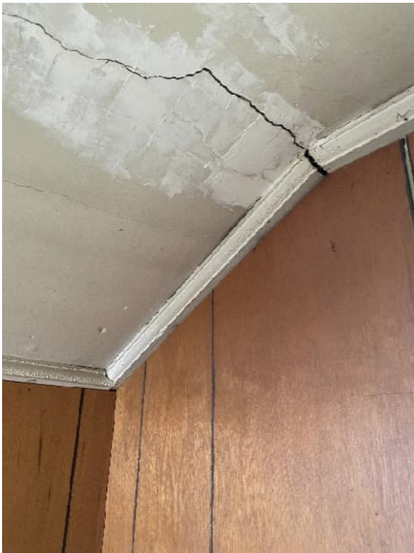
Plate 54: Cracks and repairs of southeast room
